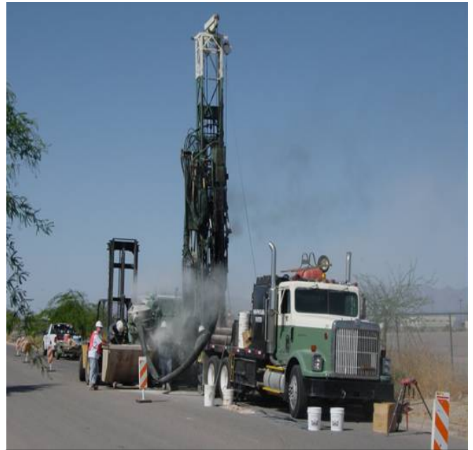
Figure 2. Drilling and installing a groundwater monitor well to evaluate the quality of groundwater.
